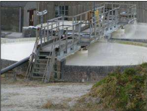
Fig 7: Large slurry tanks
