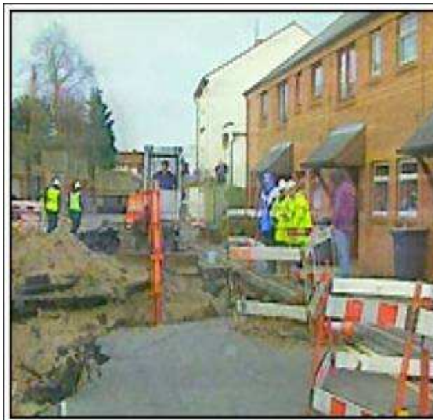
Photo from BBC news website showing damage and repair work to the houses in Field Road.
