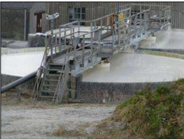
Fig 7: Large slurry tanks
